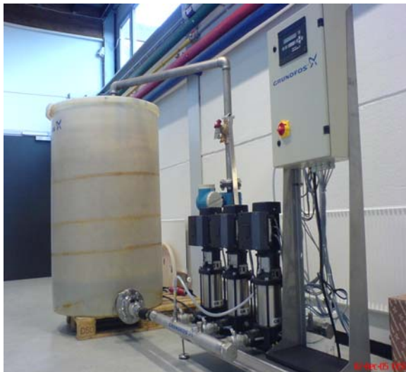
Fig.1 Grundfos set-up in AAUE
