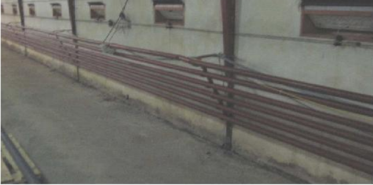
Fig.2 Outside and inside of the SKOV's testing facility in Syvsten
