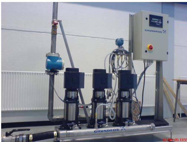
Fig.1 The lab-sized tree-pump boosting system
